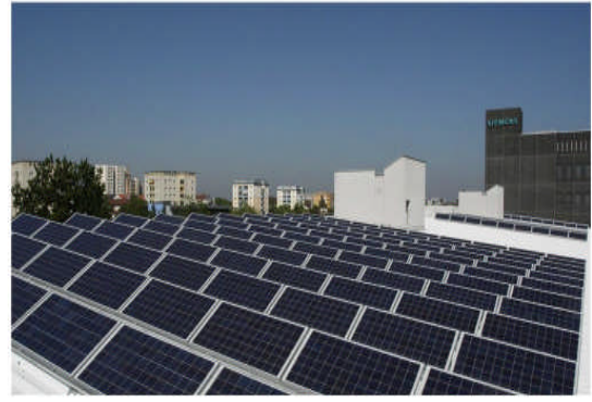
Rooftop PV (Source: Siemens)
