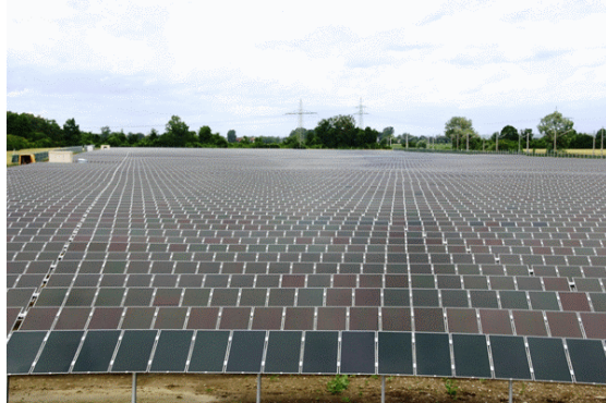
Solar Park (Source: Falcon Green Energy)
