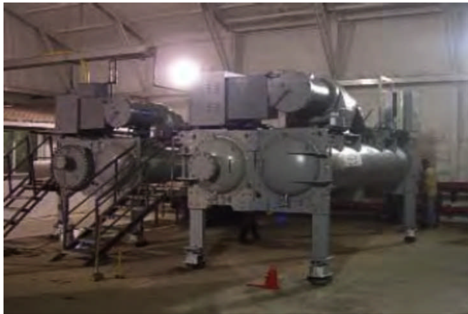
ORC #1 (background) and ORC #2 installed in the power plant building Source: Chena Power Company
